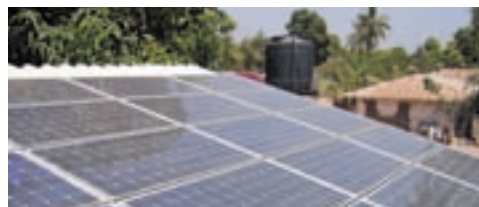
PV generator in Gambia
